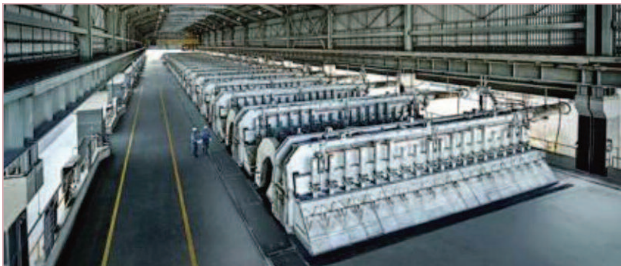
Figure 2. Typical arrangement of aluminum furnaces. An internal building configuration at an aluminum smelter.
